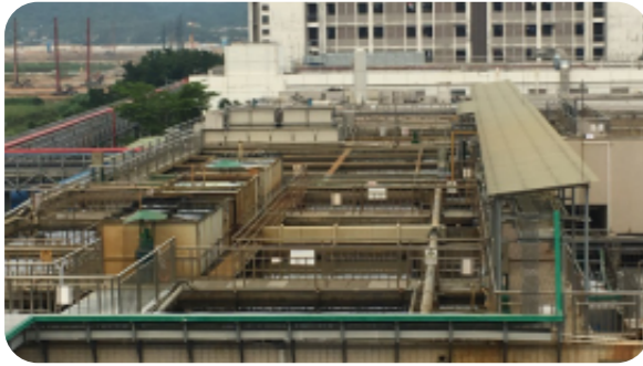
Wastewater Treatment Tank
