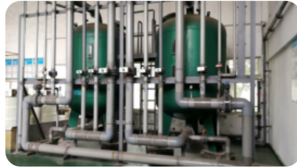
Recycled Water Reuse System
