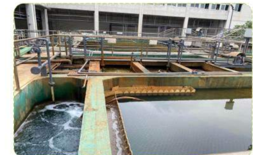
(F6 wastewater treatment system)
